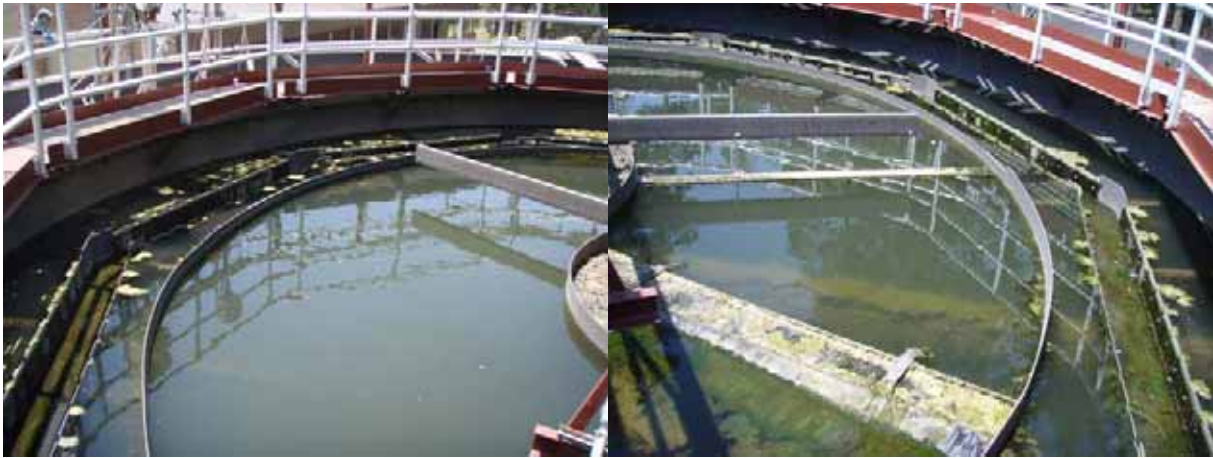
Figures 14, 15. Package treatment plant No. 2. Algae is growing on effluent troughs, scum trough, and other submerged structures. Floating algae is also growing outside of the scum ring. SMJ.
