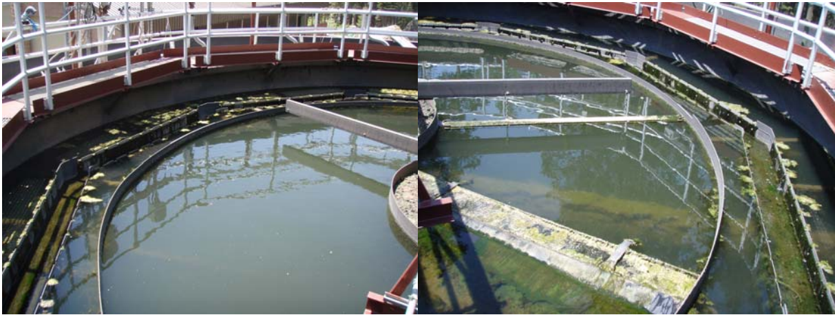
Figures 14, 15. Package treatment plant No. 2. Algae is growing on effluent troughs, scum trough, and other submerged structures. Floating algae is also growing outside of the scum ring. SMJ.
